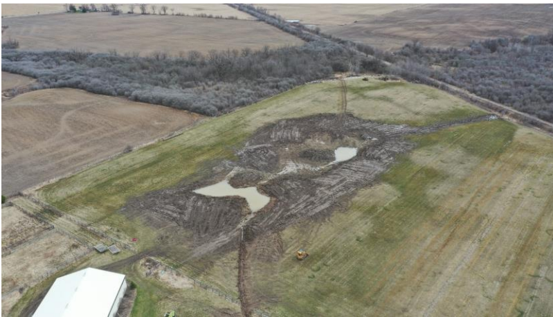
Figure 1: the Hogan wetland was completed at the beginning of April and has already started to recharge. This is the 2 nd wetland project to be established this year.
