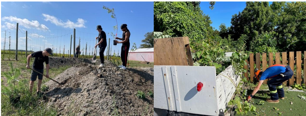
Staff & volunteers participating in restorative work at Red Barn Brewing Co. (left) and Sons of Kent Brewing Co. (right).
