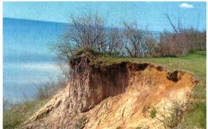
Lake Erie bluff erosion continues to present challenges to landowners and municipalities.
